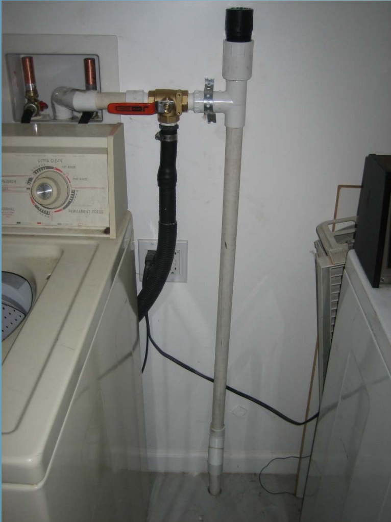
Example of indoor portion of L2L system.
