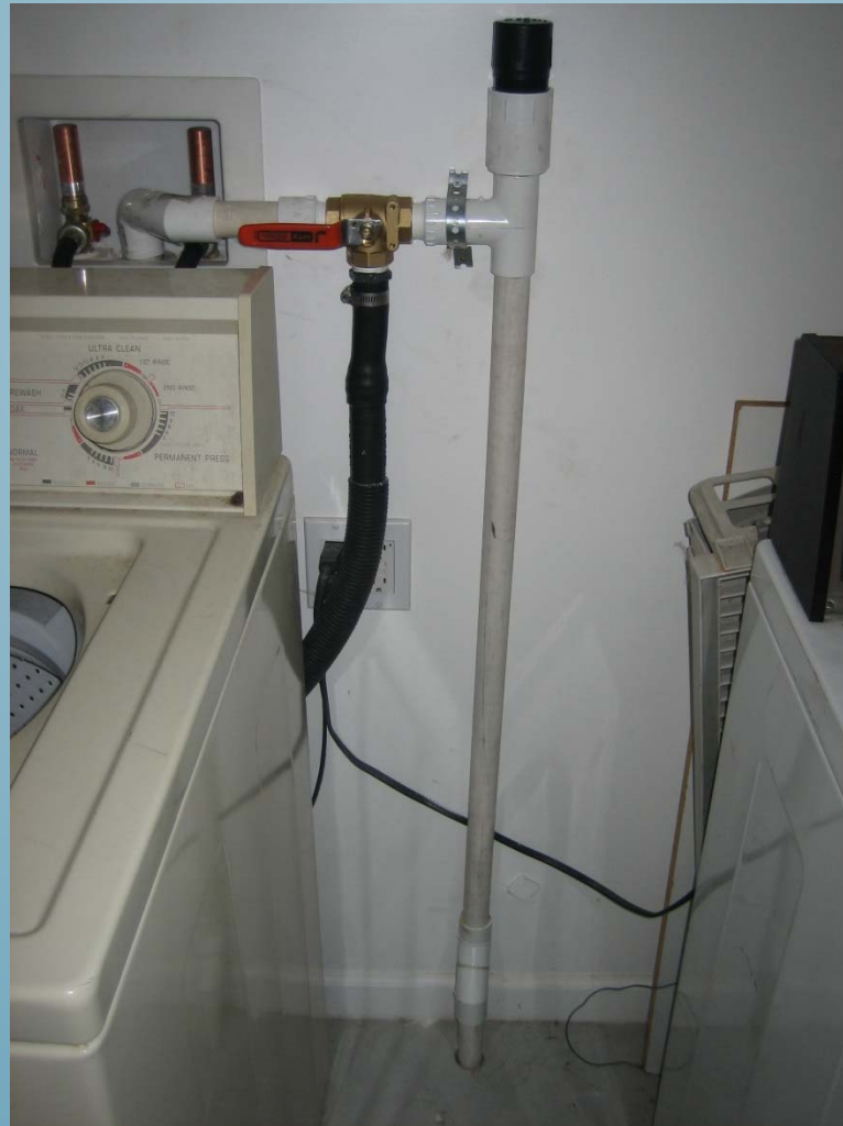
Example of indoor portion of L2L system.
