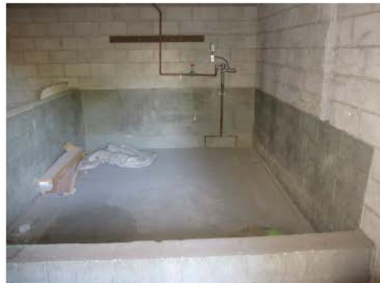
Photograph 28. Secondary containment area at JC Penney.
