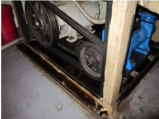
Photograph 5. Elevator equipment with hydraulic fluid in drip pan.
