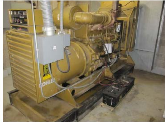
Photograph 6. One of three on-site emergency generators.
