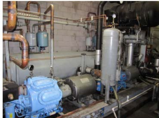
Photograph 8. Refrigeration equipment at Cupertino Ice Center.
