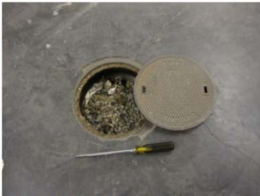
Photograph 27. Former hydraulic lift filled with pea gravel at JC Penney.
