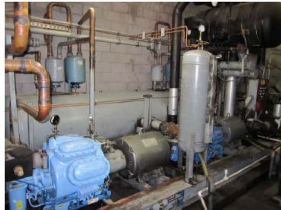
Photograph 8. Refrigeration equipment at Cupertino Ice Center.
