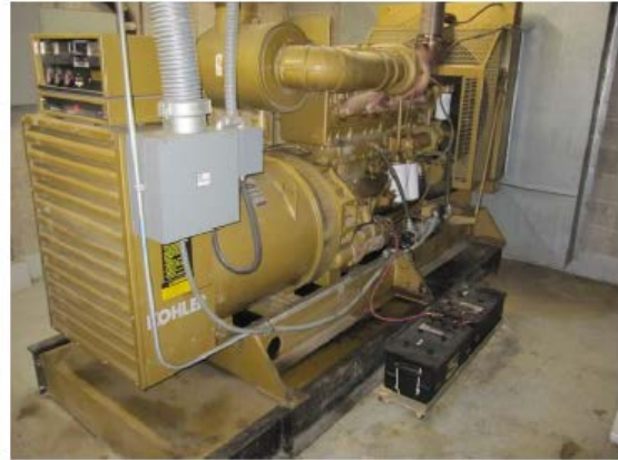
Photograph 6. One of three on-site emergency generators.
