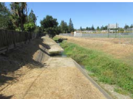
Photo 9: The existing maintenance road and ramp on the south side of the creek as it passes Wilson Park looking west. As shown in the photo, the base of the existing maintenance road/future trail is inundated with creek flows.
