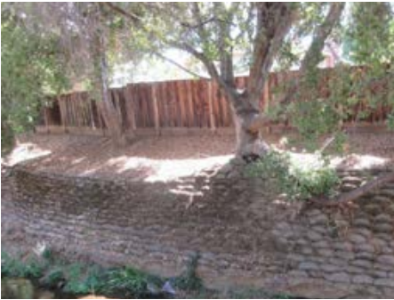
Photo 3: Rip rap stabilization of south side of the creek, south of Rodrigues Avenue.
