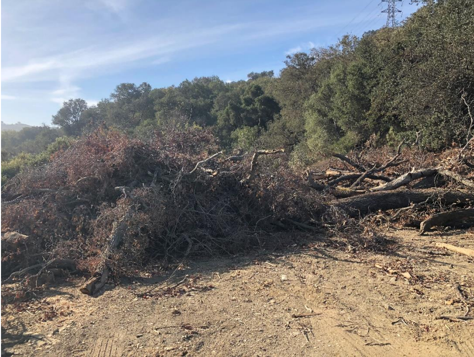
View of the primary debris pile.
