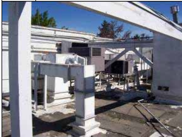
9. Roof mounted heating and air conditioning equipment
