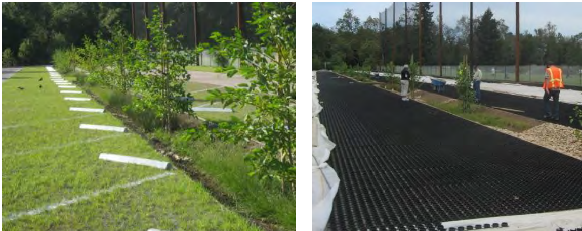
Figure 2-10 Completed green parking bays (above left) and parking bays under construction, showing the recycled plastic geocells that support vehicle weight (above right). (Source: City of Cupertino)
