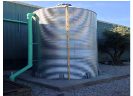
Figure 2-8 Rainwater harvesting cistern, Environmental Innovation Center, San José (Source: City of San Jose)
