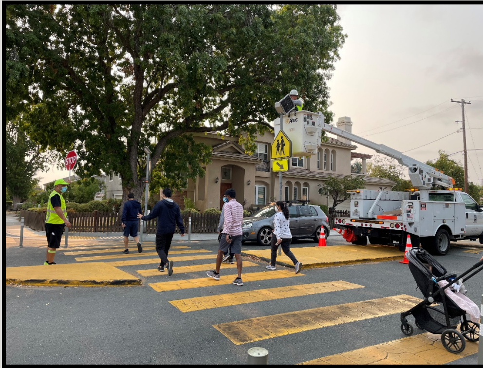
RRFB Installation at Sedgwick: Tantau and Barnhart
