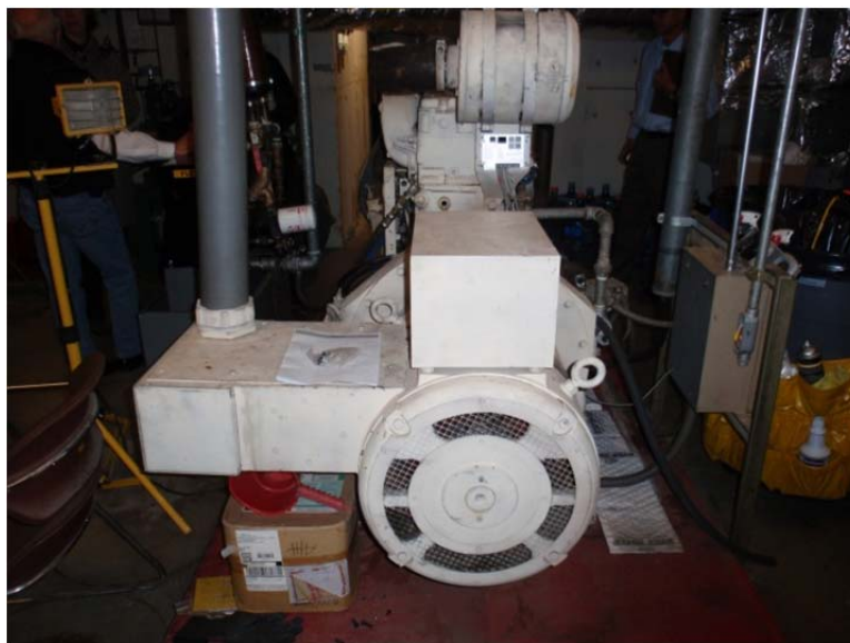
Figure 5G (Indoor Generator)
