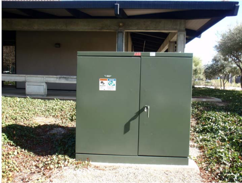
Figure 1E (PG&E Transformer)
