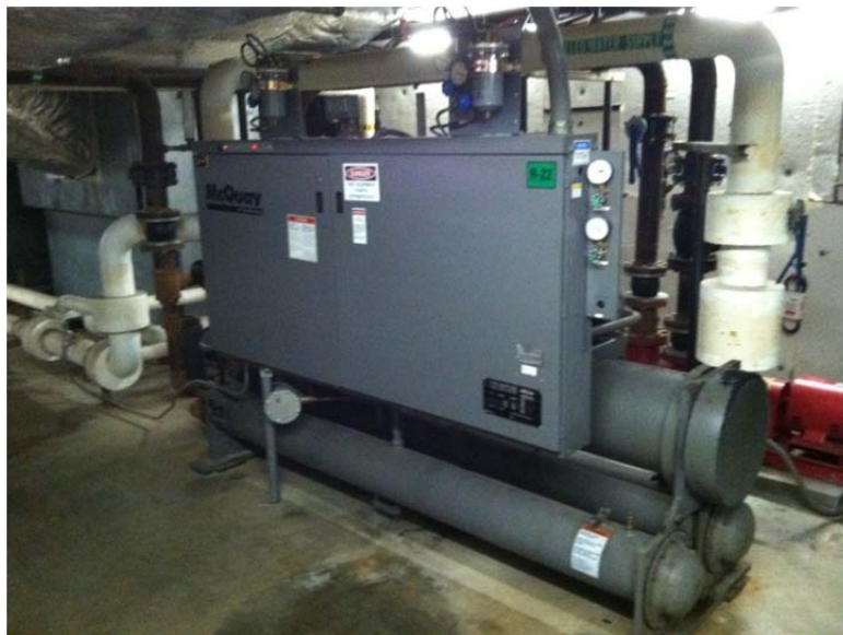
Figure 5B (Water-cooled 70 Ton Chiller)
