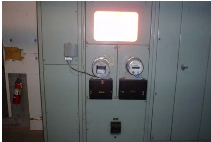
Figure 5F (Main Switchboard)
