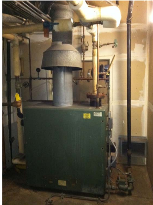
Figure 5C (Gas Fired Boiler)
