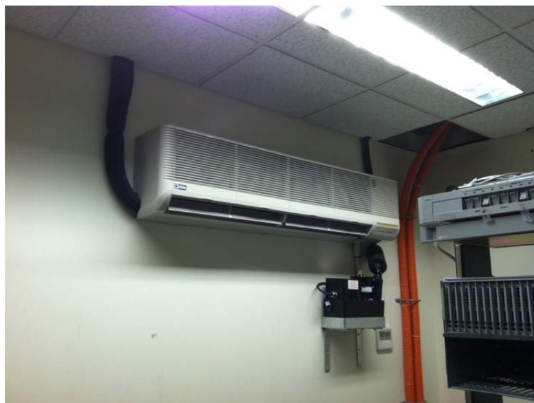
Figure 5D (Server room AC unit (1 of 2))
