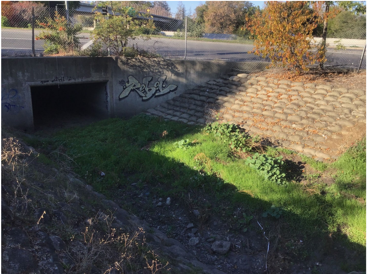
Photo 5. The Junipero Serra Channel, between Wolfe Road and Calabazas Creek, is a vegetated engineered earthen channel.
