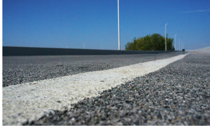
Improve pavement friction
