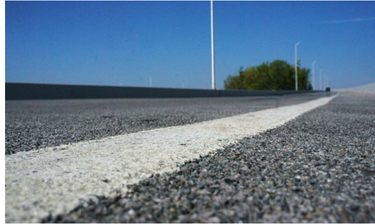
Improve pavement friction
