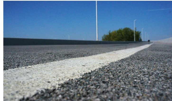
Improve pavement friction
