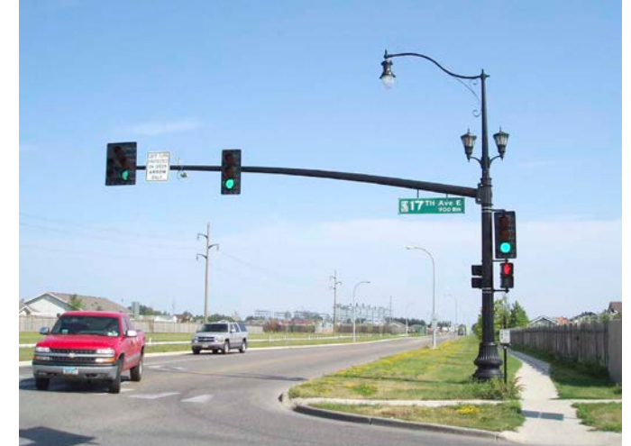
Convert signal to mast arm
