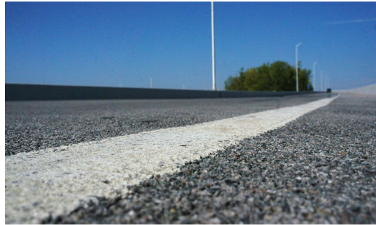
Improve pavement friction
