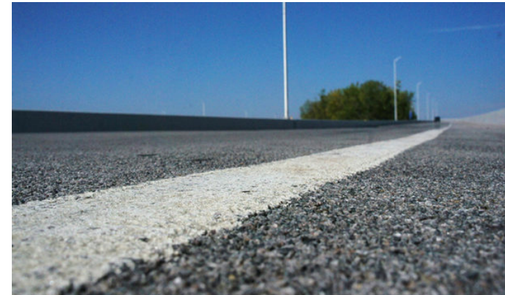
Improve pavement friction
