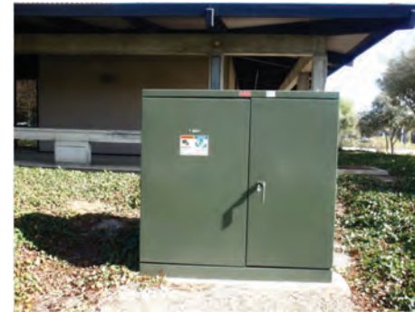
Figure 1E (PG&E Transformer)
