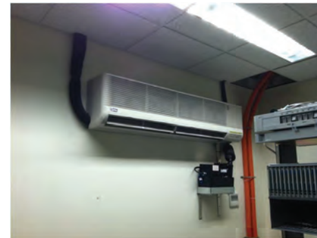
Figure 5D (Server room AC unit (1 of 2))
