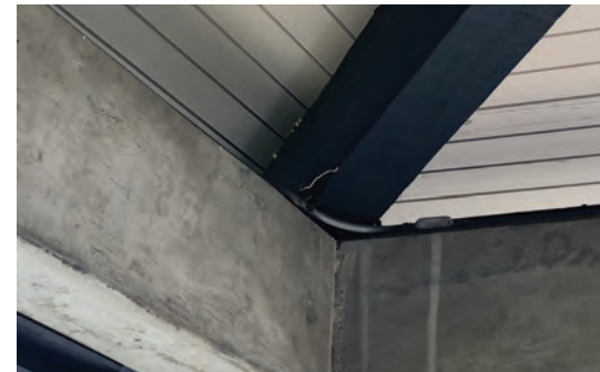
Crack in Beam
