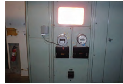
Figure 5F (Main Switchboard)
