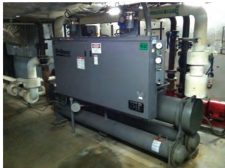
Figure 5B (Water-cooled 70 Ton Chiller)
