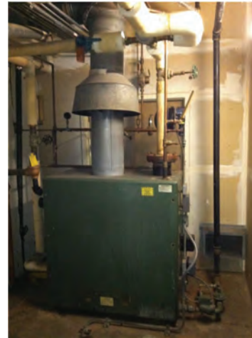
Figure 5C (Gas Fired Boiler)
