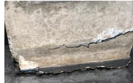
Additional Cracking at Column Base
