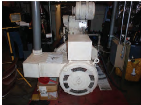
Figure 5G (Indoor Generator)
