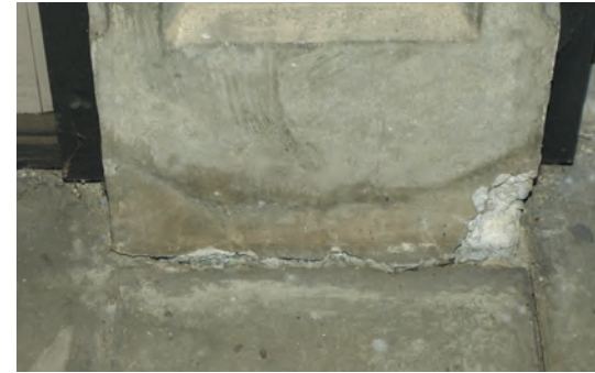
Cracking at Column Base
