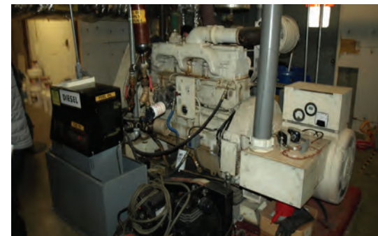
Diesel Generator Inside Building
