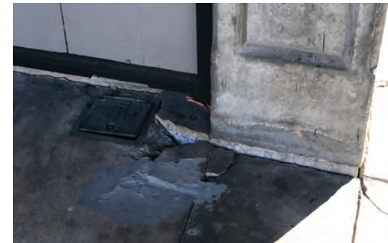
Crack in Column and Settlement
