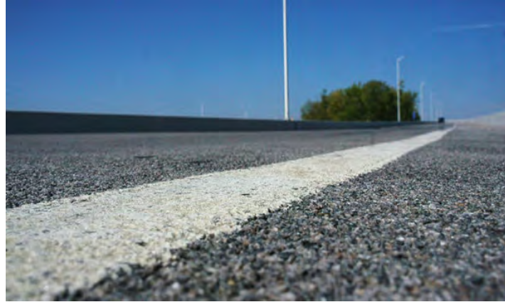
Improve pavement friction
