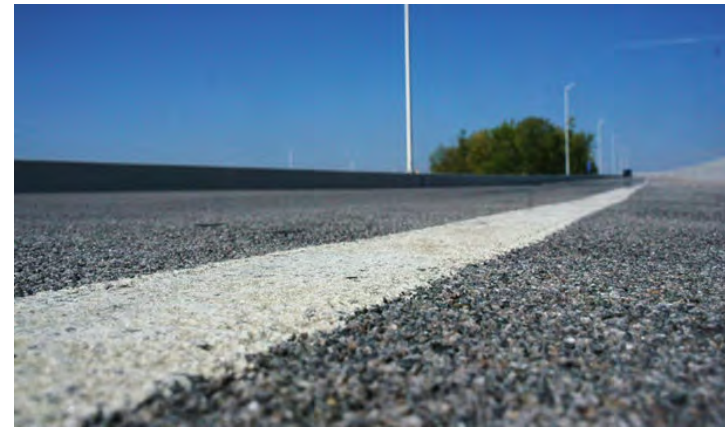
Improve pavement friction
