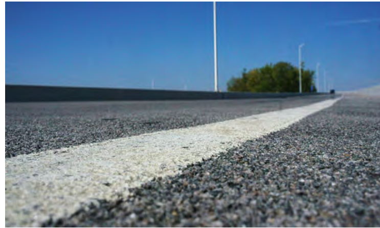
Improve pavement friction
