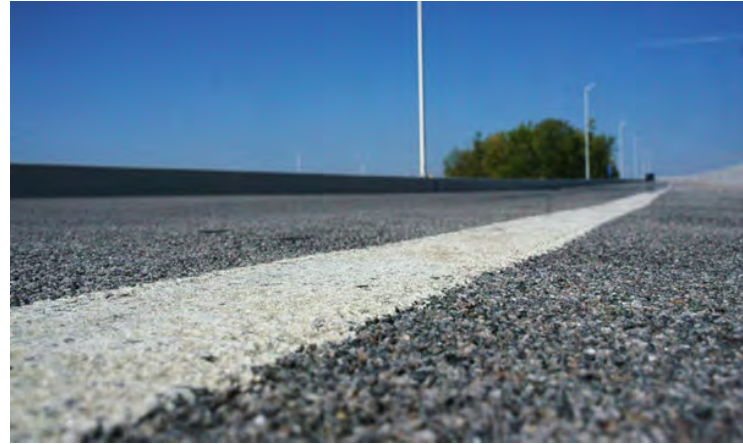
Improve pavement friction
