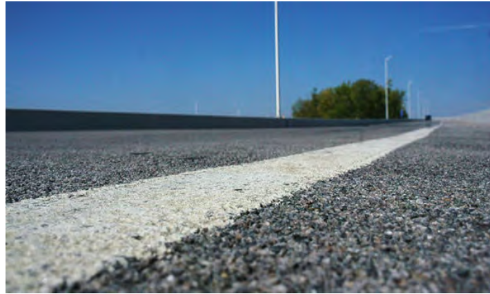
Improve pavement friction
