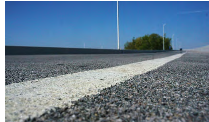
Improve pavement friction
