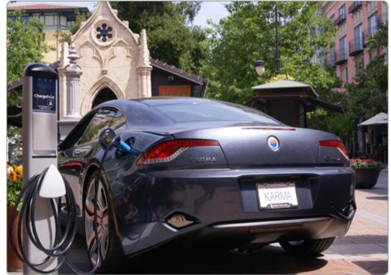
EREV charging at Level II w J1772
