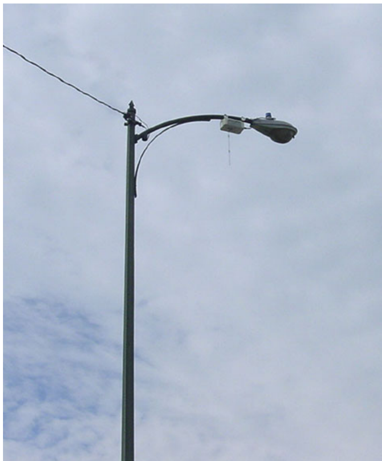
(Personal wireless facility at Swallow Drive and Lorne Way, Sunnyvale, CA)
