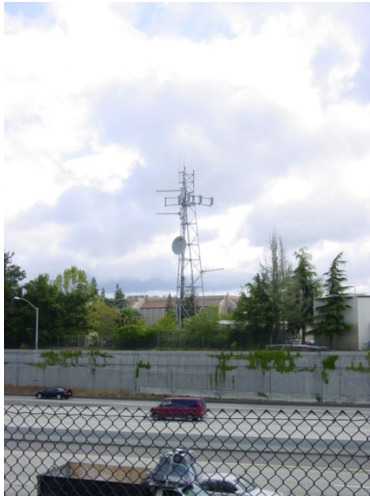
(Antennas mounted on a lattice tower. Site located at De Anza College near Highway 85.)
