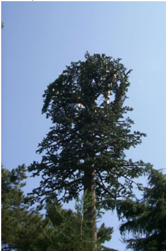
(Treepole style antenna mount located on San Tomas Expressway near its intersection with Hamilton Avenue, Campbell, CA.)
