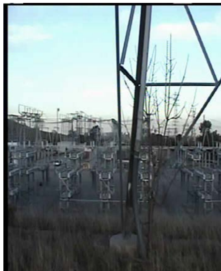
(Depicted are cables enclosed in a conduit that runs along the leg of a lattice tower located above the Monta Vista electrical substation in Cupertino, CA.)
