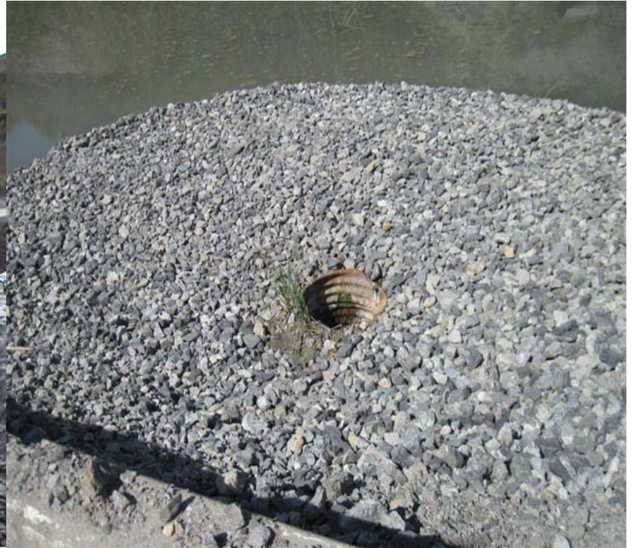
Pond 9 – discharge w/ water polishing limestone filter
