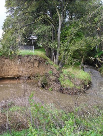
Erosion may result from increases in the amount and rate of runoff entering a creek.
