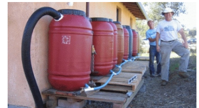
Rain barrel system
