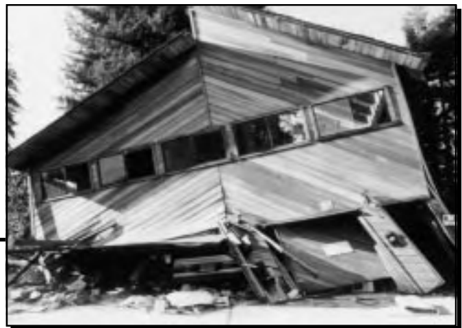
This mountain home was built over a garage, and its walls were not strong enough to withstand an earthquake.
