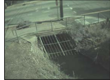
Photo 7a: Trash Rack in Morgan Hill
