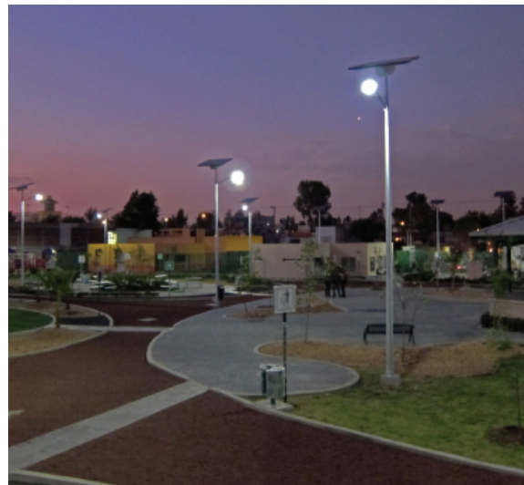
LED and solar-powered lighting is an important way to reduce energy costs while also creating a safe pedestrian environment at night
